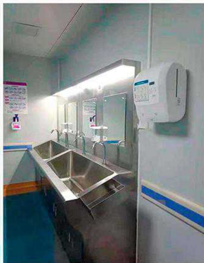
Infrared Induction Hand Washing Basin
