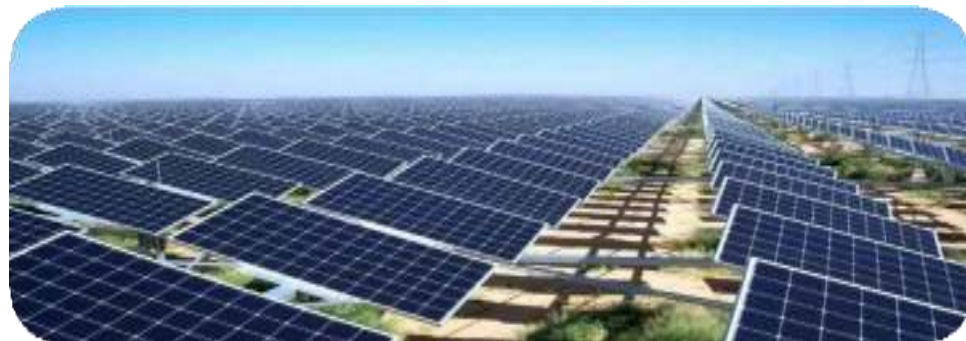
Power Generation Panel
