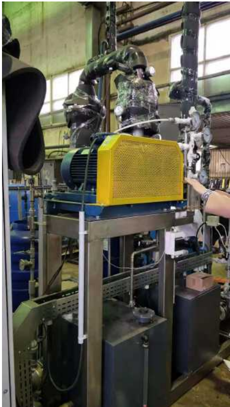
HDSR80, steam compressor
