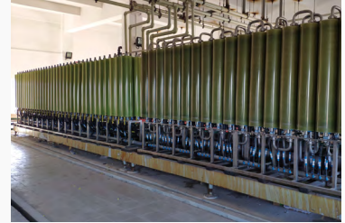
Guangdong Desulfurization Wastewater 48t/h
