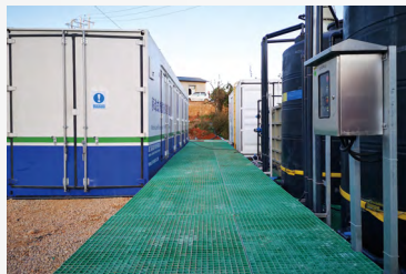
Yunnan Landfill Leachate 200t/d
