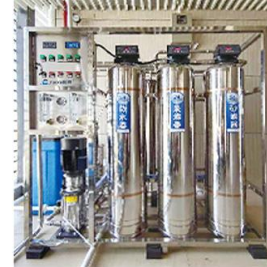
Guangzhou Development Zone Middle School Water Purification Project
