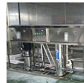
Beijing Jingdiao Branch Reverse Osmosis + EDI
