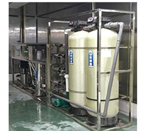
Huizhou Electronics Factory Pure Water Equipment
