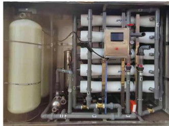
8T/H RO unit
