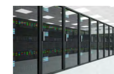
High heat density data center
