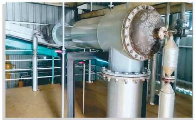
STEAM JET VACUUM SYSTEMS
