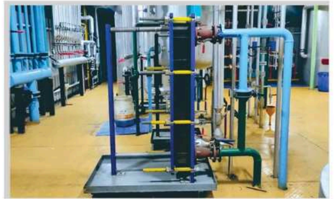
PLATE HEAT EXCHANGER
