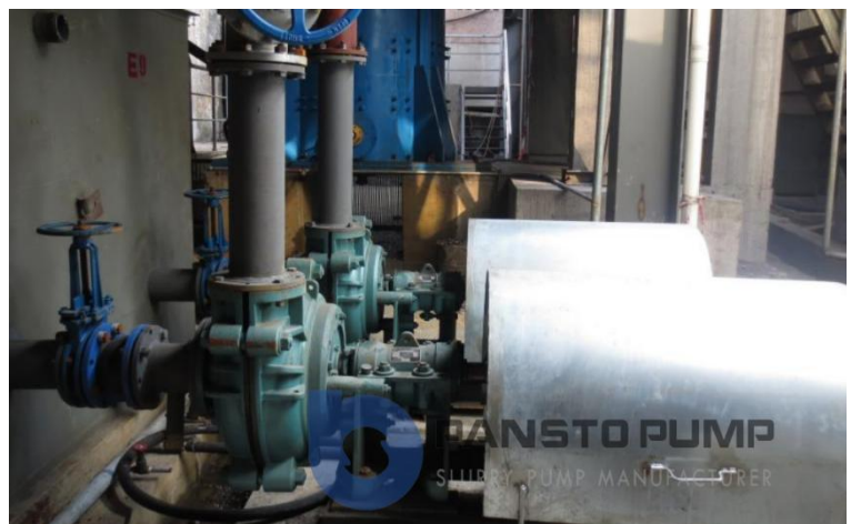
PH pumps are used in Copper Concentration Plant, Africa
