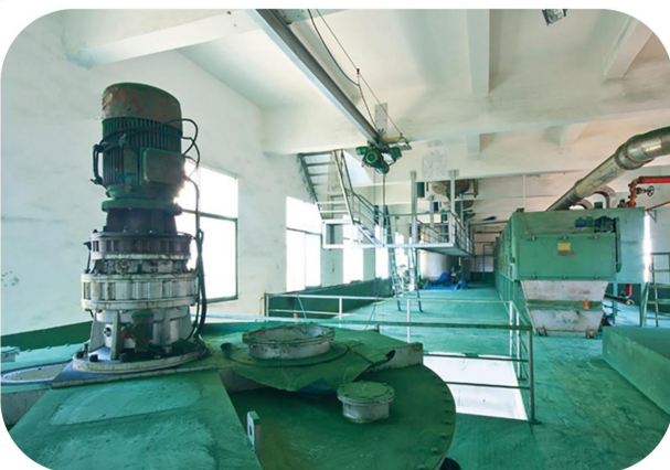
氧化铁绿生产车间 THE COMPANY EQUIPMENT(COMPOUND GREEN)
