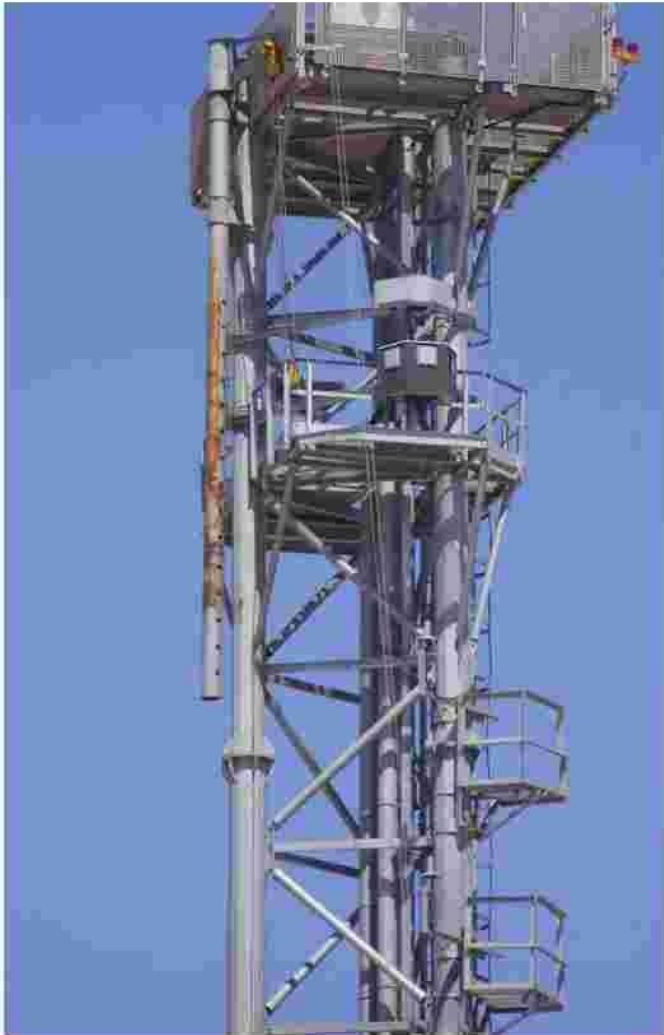
17m 3-LEG RADAR TOWER
