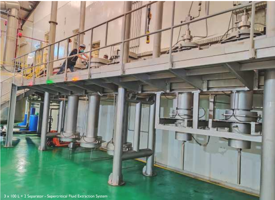
3 x 100 L + 2 Separator - Supercritical Fluid Extraction System
