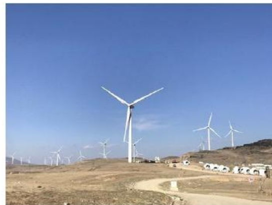
Yunnan Qiaojia County Xinchanggou Haiba wind farm project
