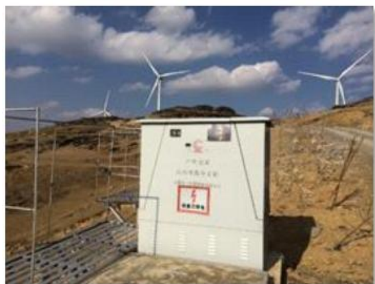
Yunnan 49.5MW Qiaojia Dalai Shishan Wind Farm project
