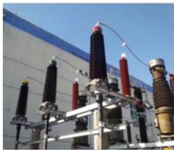
Linqi 110kV substation, Anyang, Henan
