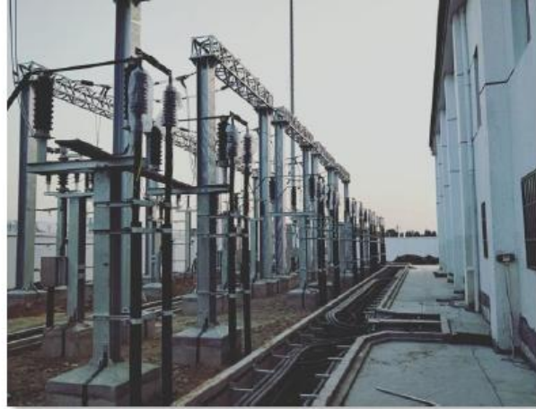
Lianyungang Substation of Qinglian Railway
