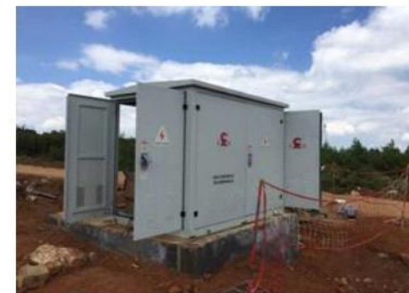
Qujing City, Yunnan Province Huaneng Fuyuan Guangliangzi Wind Power (Phase II) project
