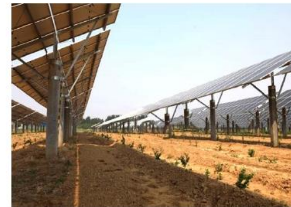
Henan Nangong photovoltaic power station project
