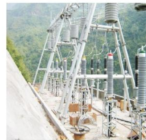
Malutang Power Plant, Wenshan City, Yunnan Province Phase II 220kV cable project
