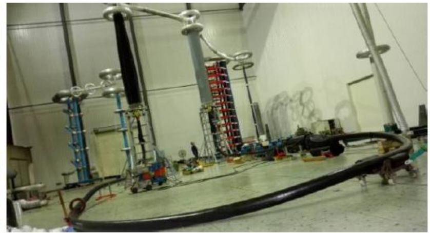
500kV cable and accessories test circuit
