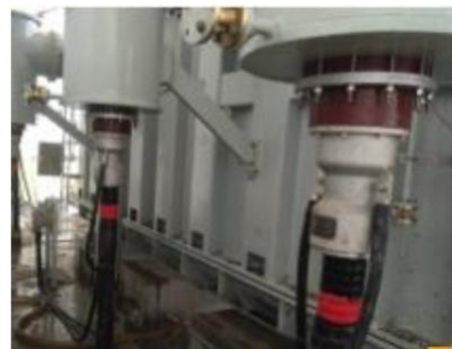
Hubei Wuhan Taojialing 220kV power transmission and transformation project
