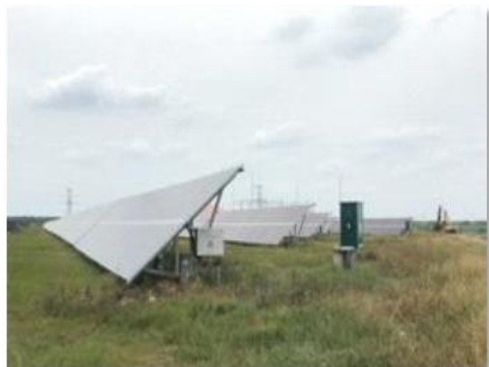
Anda Shengping photovoltaic power station project in Heilongjiang Province
