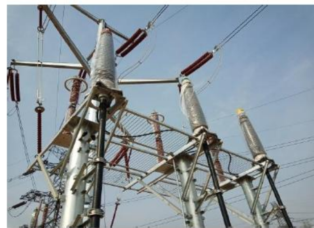
Zhaojialiu 220kV traction station power line project
