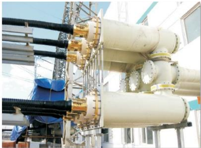
Inner Mongolia Baotou Aluminum Plant three series high-tech double line 220kV cable project
