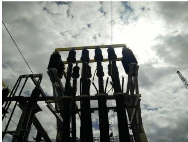
27.5kV Kunming Hub Project
