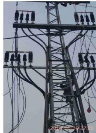
27.5kV Shanghai-kunming high-speed Railway
