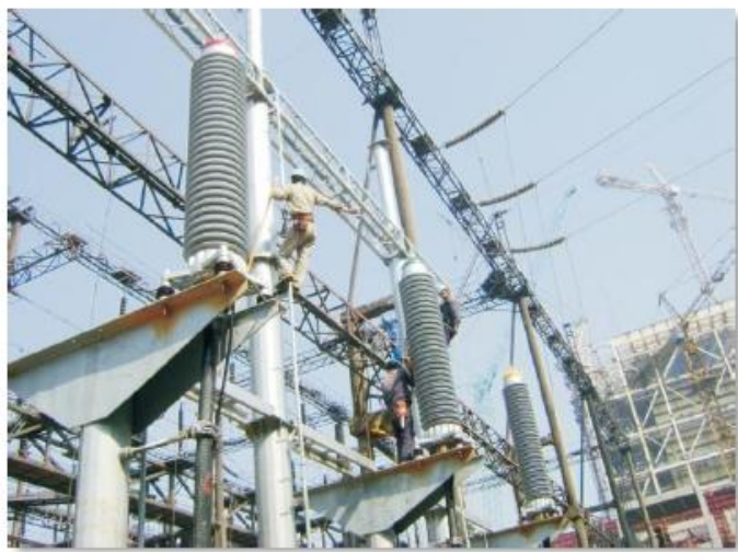
Nanjing Hualian thermal Power Plant 220kV cable
