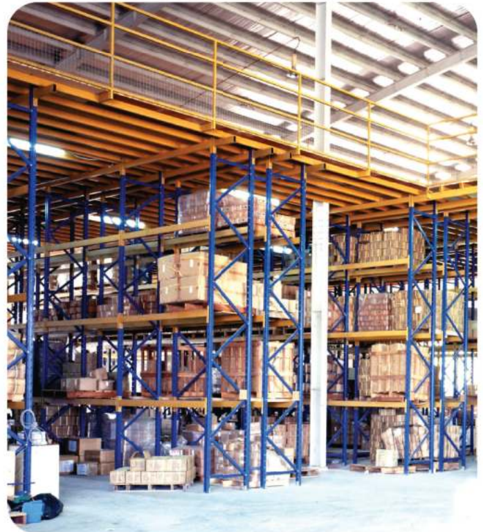
Rack Supported Platform
