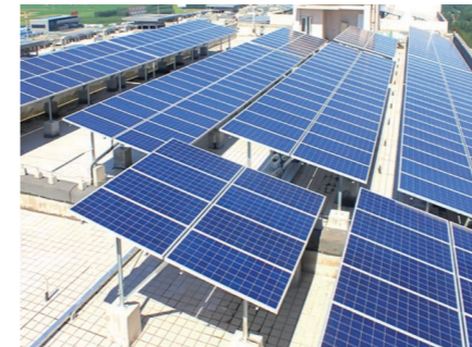
光伏储能/Photovoltaic Energy Storage
