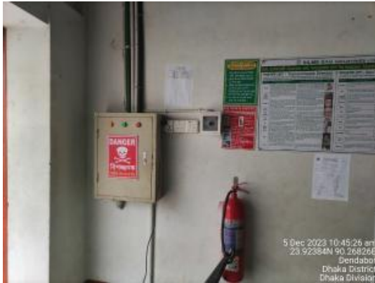
Electrical distribution board.jpg
